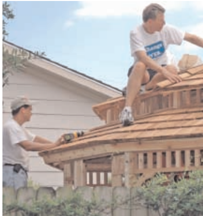
Enbridge employees Terry Register (left) and Dave Agerton (right) put the finishing touches on an outside reflection space for residents.
