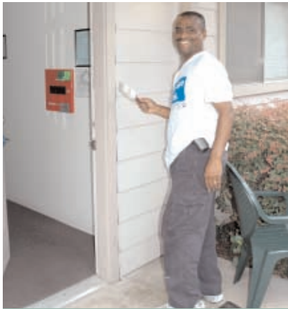
Enbridge employee Anthony Brown adds a fresh coat of paint to one of the transitional homes.
